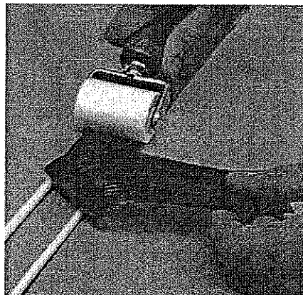
Figure 2 - Place weatherstrip into silicone and seat UltraSpan US1100 silicone weatherstrip using a roller.
