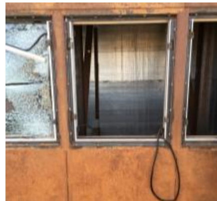
Figure C.30: Specimen 3-1 Post-Blast Condition
