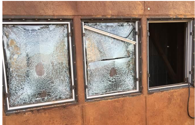
Figure C.26: Specimen 2-3 Post-Blast Condition
