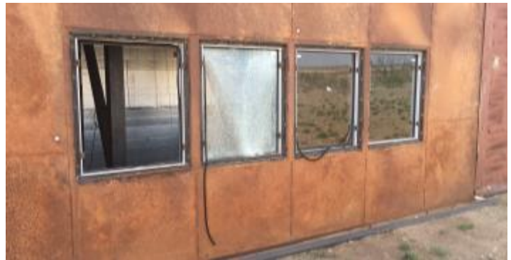
Figure C.34: Specimen 3-3 Post-Blast Condition
