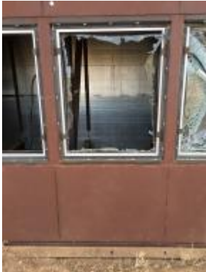
Figure C.11: Specimen 1-3 Post-Blast Condition
