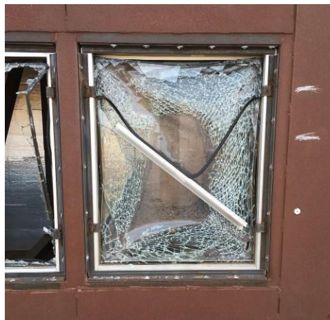
Figure C.16: Specimen 2-1 Post-Blast Condition
