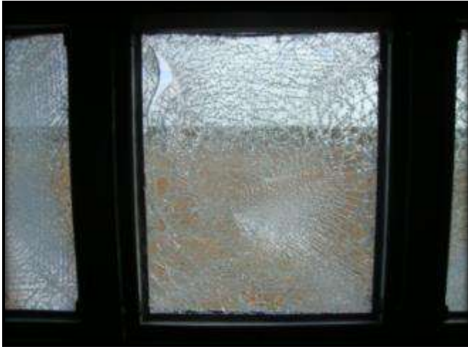
Figure C.17: Specimen 11 Internal Post-Blast Condition
