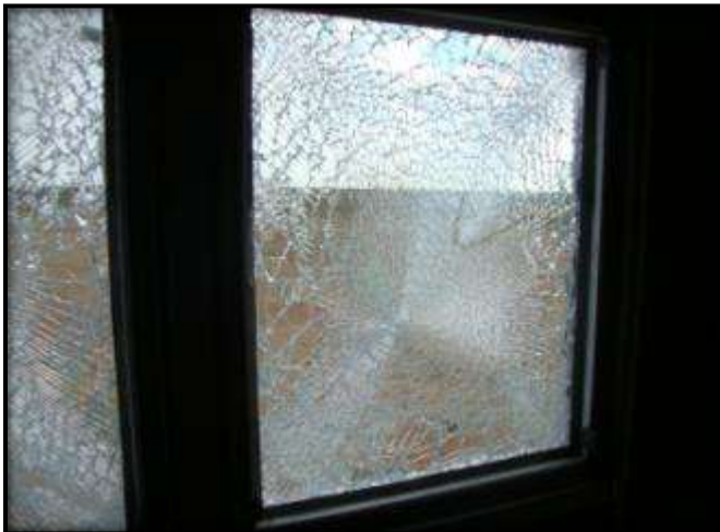
Figure C.15: Specimen 9 Internal Post-Blast Condition
