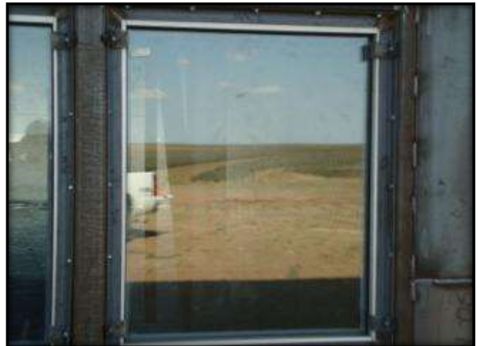
Figure C.26: Specimen 16 External Post-Blast Condition
