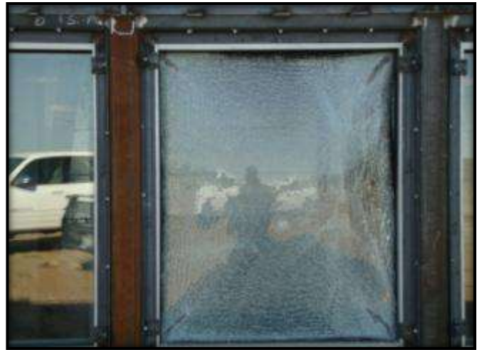
Figure C.24: Specimen 14 External Post-Blast Condition
