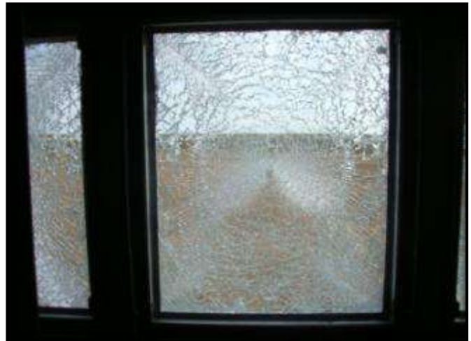
Figure C.16: Specimen 10 Internal Post-Blast Condition
