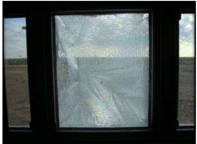
Figure C.28: Specimen 14 Internal Post-Blast Condition
