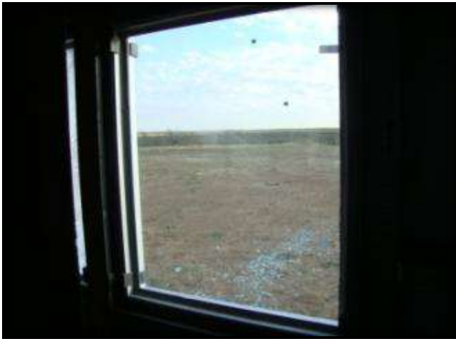
Figure C.27: Specimen 13 Internal Post-Blast Condition
