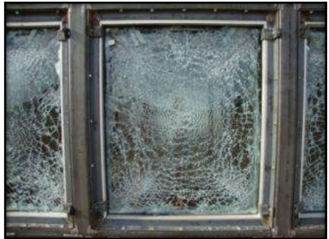
Figure C.12: Specimen 10 External Post-Blast Condition
