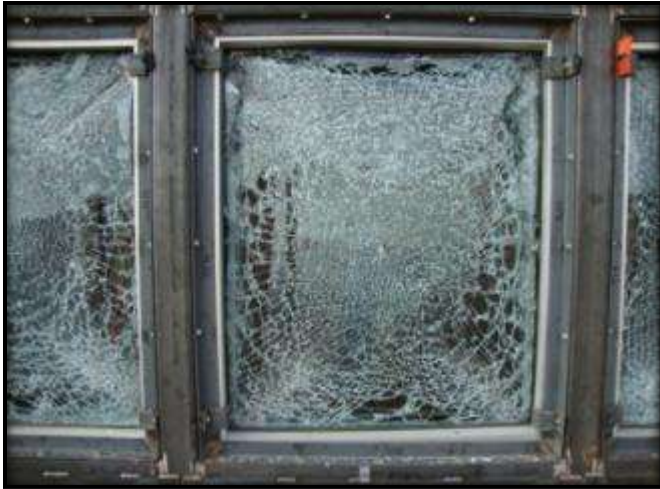
Figure C.13: Specimen 11 External Post-Blast Condition
