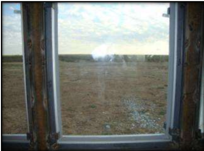
Figure C.29: Specimen 15 Internal Post-Blast Condition
